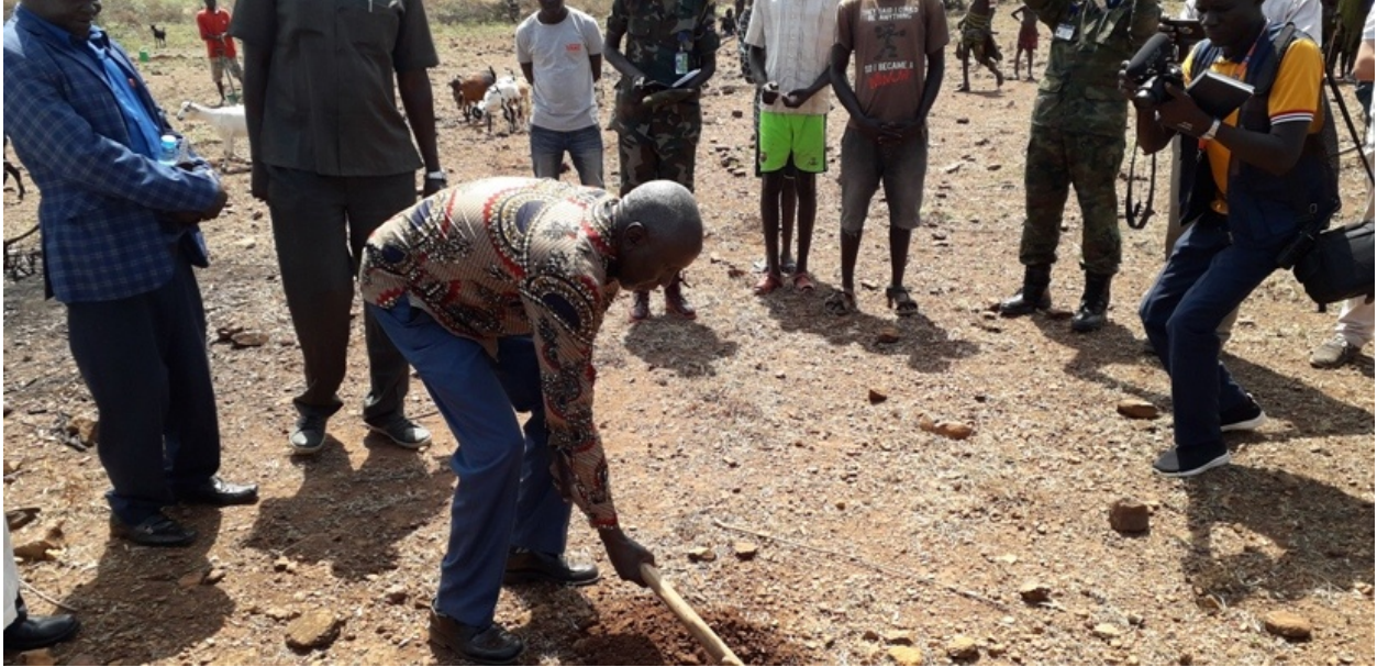
Deputy Governor of Former Kapoeta State, South Sudan, officially opens the construction site by ground breaking action of digging the foundation
