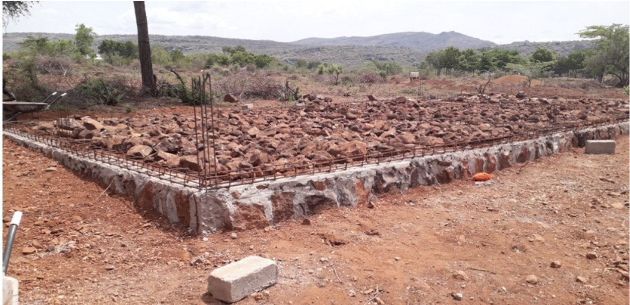
On-going Construction of two classrooms and office space for St. Thomas Secondary School
